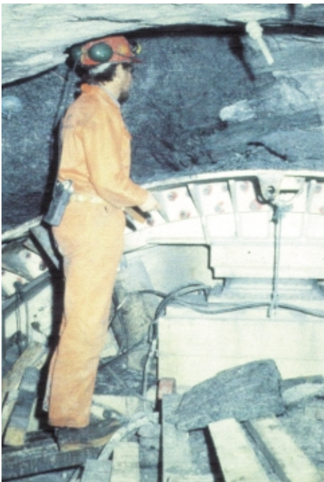
Fig. 4 Rock spalling overbreak in roof
