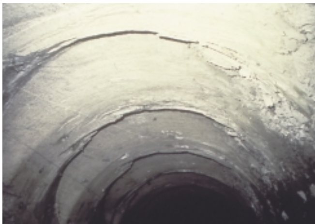
Fig. 2 Overbreak due to crushing and spalling
