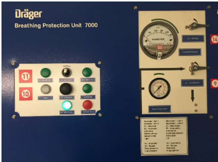
Figure 6-23: the BPU-control panel.
