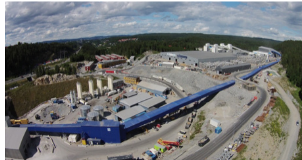
Figure 9-2: An overview of the rig area with conveyor belt (blue covered), which brought all excavation material from the tunnels up to the upper rig area, close to the deposit area.
