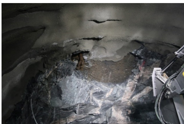
Figure 11-8: The exposed concrete plate from below.
