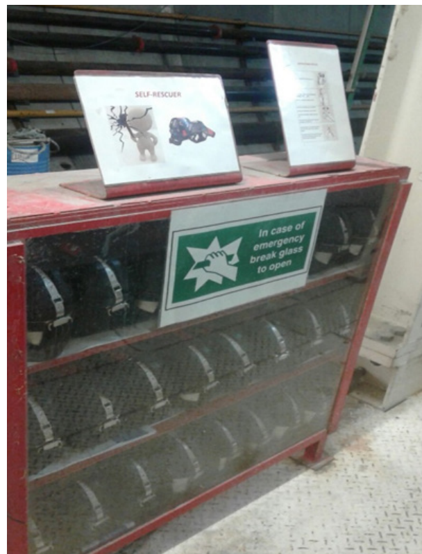
Figure 6-16: Self-rescuer stored in the TBM back up.
