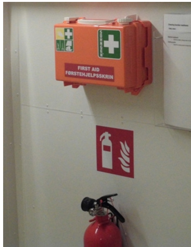
Figure 6-26: First aid and fire extinguisher.
