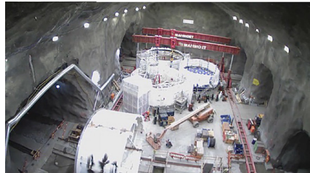
Figure 12-7: Northern cavern with the jacking system used for the assembly of the TBMs Euphemia and Ellisiv.
