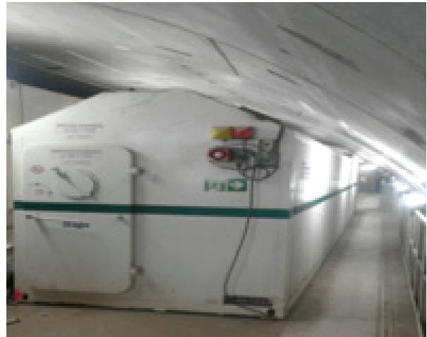
Figure 6-19: Gas detector in the refuge chambers.
