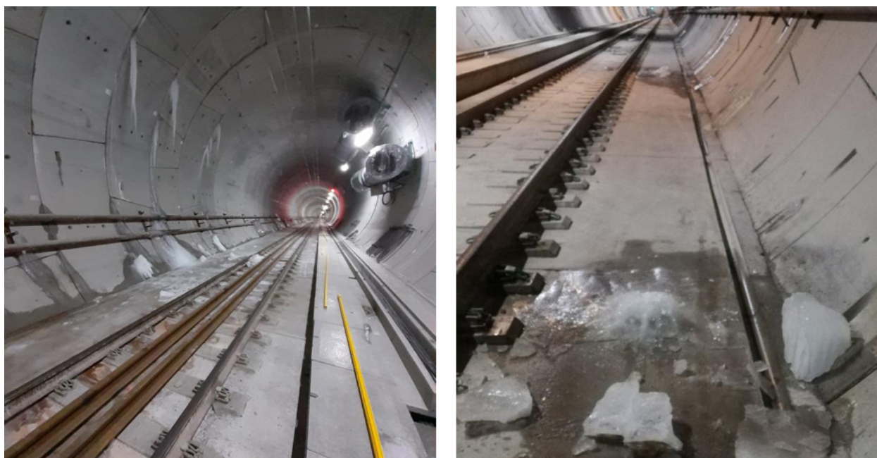
Figure 18-3: Ice formations in the tunnel.
