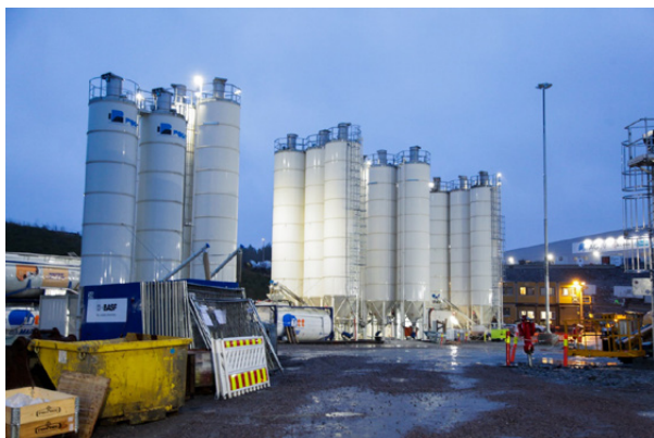
Figure 16-22: The bi-component plant located at the rig area outside the tunnel portal.
