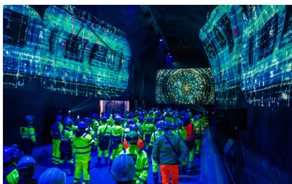
Figure 12-19: Double breakthrough in the north, where the two machines arrived into two parallel caverns. Photo: Nicolas Tourrenc.
