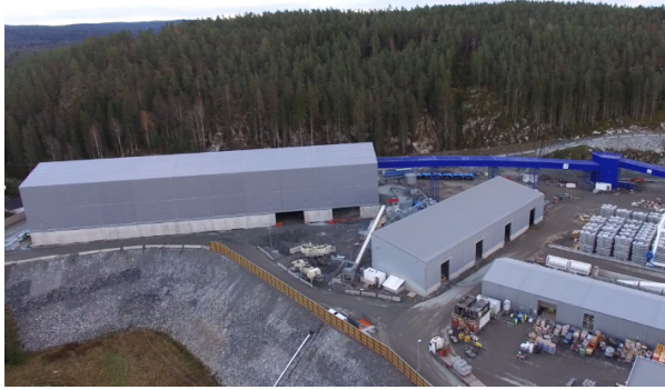
Figure 12-4: The spoil shed (large building) with the conveyor belt (blue) and the building for storage of aggregates (four openings).
