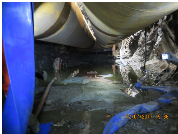
Figure 11-7: The exposed invert of the Alna River tunnel under the steel pipes.
