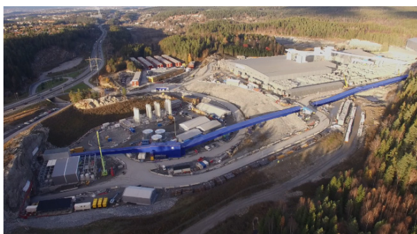
Figure 12-12: An overview of the site. In blue, alignment of the fully covered conveyor belt from the portal of the northern access tunnel towards the spoil area.
