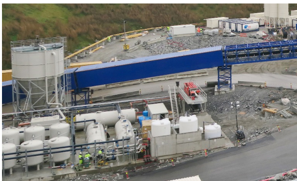
Figure 12-14: One of the two water treatment plants.
