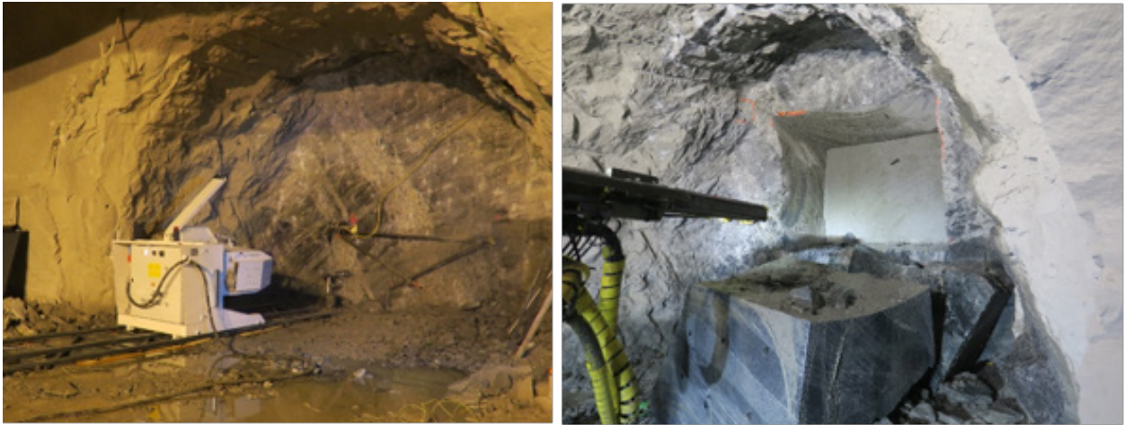
Figure 13-10: Careful blasting, drill and split and finally wire cutting from the escape tunnel.
