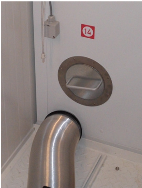
Figure 6-25: Outlet for fresh air.
