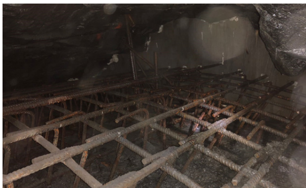
Figure 11-20: The missing concrete in the crown of Midtgardsormen.
