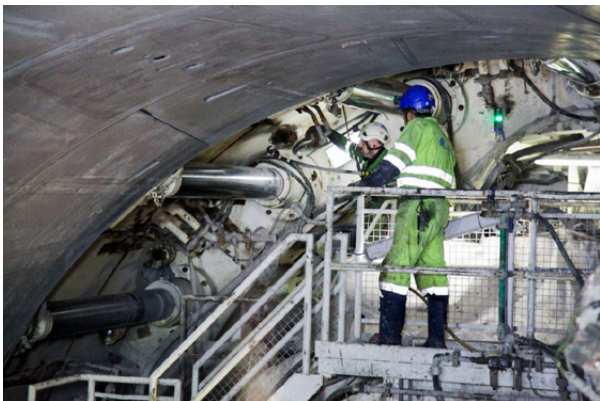
Figure 16-18: The cylinders at the TBM pushed against the segments during the installation.
