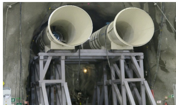
Figure 12-15: The main fans in the southern cavern.
