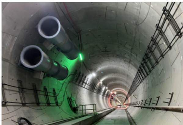
Figure 19-6: Jet fans for longitudinal ventilation.
