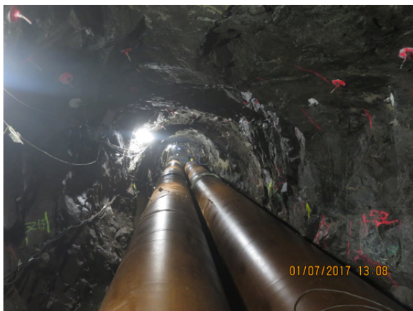
Figure 11-6: The steel pipes installed above the crossing with Inbound and Outbound Follo Line.
