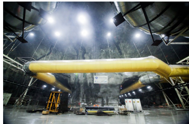
Figure 6-35: Ventilation duct in the assembly chambers.
