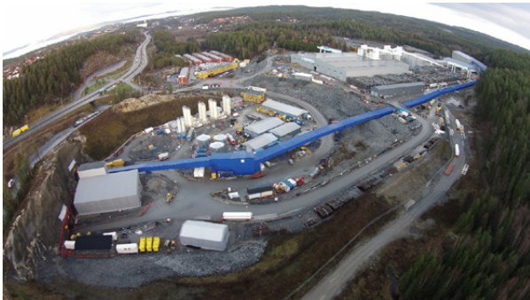
Figure 10-7: An overview of the centrally located rig area at Åsland with the conveyor belt (blue), segment factory, offices, and accommodation for the workers.
