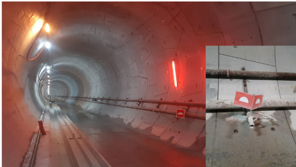
Figure 6-14: Hydrant connections in the tunnels marked with red lights.
