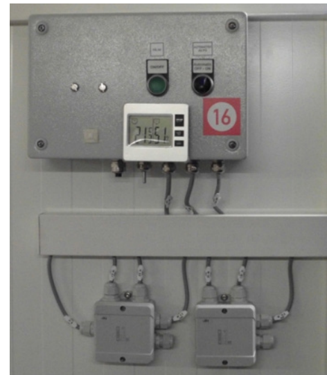
Figure 6-24: Control unit for air-cooling.
