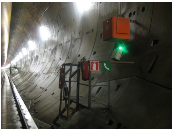
Figure 6-15: Safety point in the tunnels were marked with green lights.
