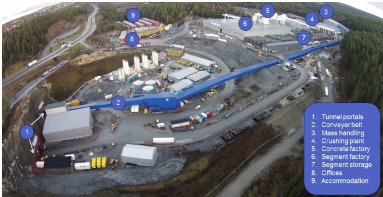
Figure 2-6: One large and efficient rig area for the operation of four TBMs including the production of the segments for the tunnel lining.
