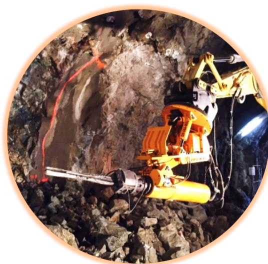
Figure 11-4: Illustration of the drilling pattern for drill and split and the hydraulic jack.
