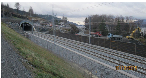
Figure 3.8.4. From the IC Dovrebanen Railway project, good quality rock used for ballast.
