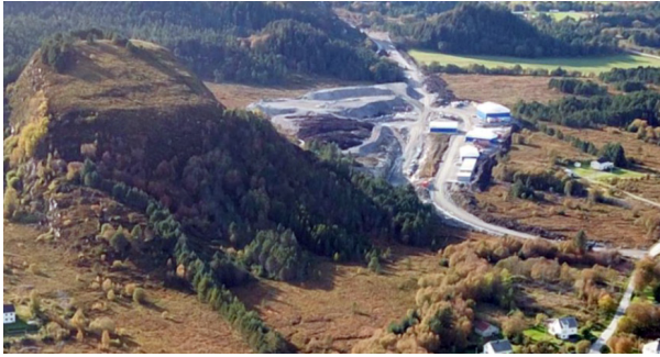
Figure 3.5.2. The building and construction area by the Fjørtoftfjord tunnel seen from the east. Ramsberget to the left in the picture. If nesting was to be registered with the owls in Ramsberget, it should not be crushed or carried out similar noisy activity in area during the period March 15 to July 15.
