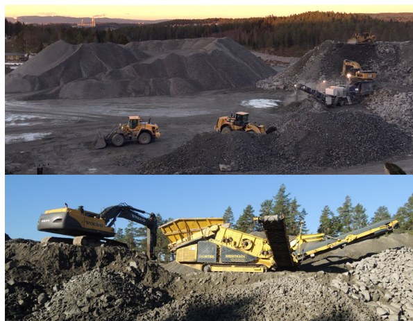
Figure 3.8.7. Stationary and mobile rock mass processing plants at the Follo Line Railway Project (B. Gammelsæter).
