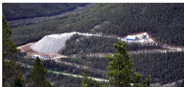
Figure 3.8.8. Tunnel muck is a valuable resource, here dumped right outside the access opening to an underground hydropower project (Photo Ø.Fæhn).
