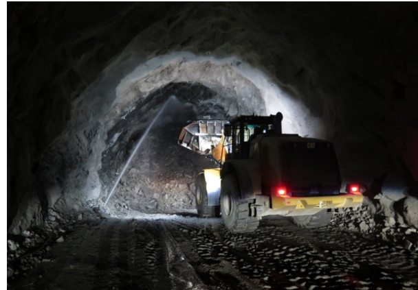
Figure 3.8.1. Loading of tunnel muck at the Rosten HEPP, Norway. (Photo Ø. Fæhn).
