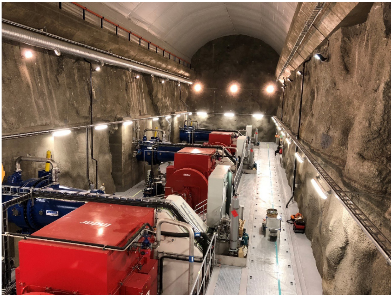
Figure 2.2.1: Storåselva Hydropower Plant the first Ceequal certified construction project in Norway.
