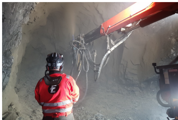
Figure 4.3.3. Using low-carbon shotcrete as the first project in Norway on a major scale (Photo: Skanska).
