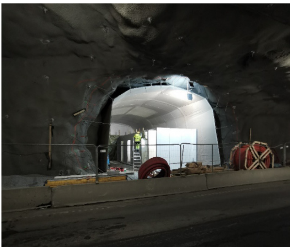
Figure 4.4.1. A technical room in a tunnel in Norway mounted without the use of heavy machinery.
