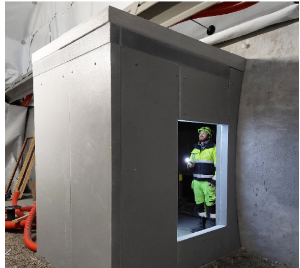
Figure 4.4.4. An emergency station made from Foamrox elements mounted behind the tunnel vault.
