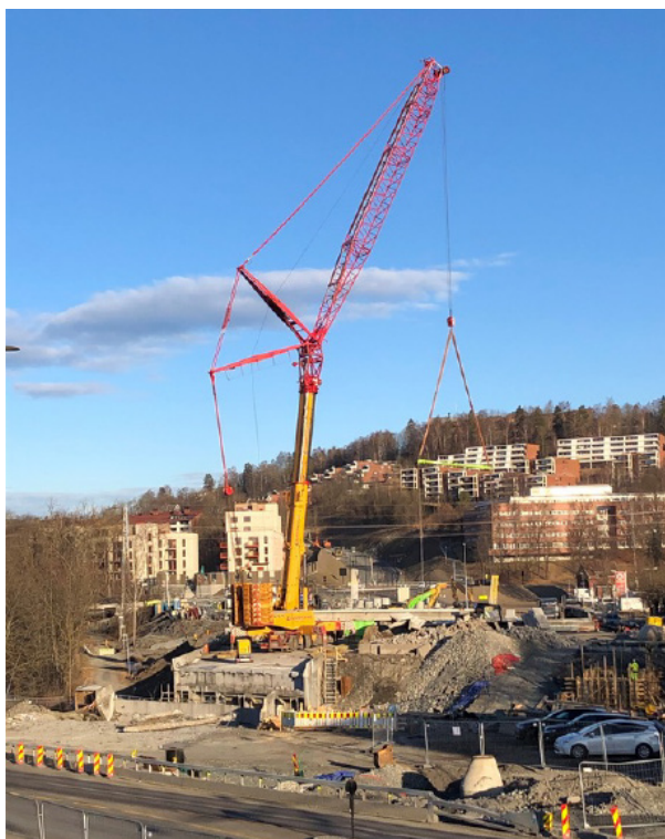
Figure 4.3.10. Dismantling: The Birkheim bridge is carefully taken apart so it can be lifted out in one piece.
