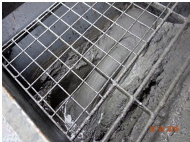
Figure 4.11 Correctly mixed grout in a mixing vessel for a grout pump. Photo Terje Kirkeby
